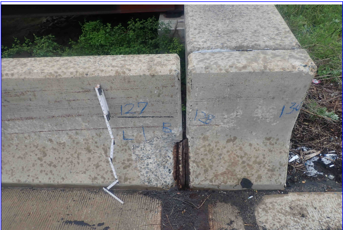
20. SPAN 3 N RC RAIL ~127-128 FT FROM W END PITTED BAR & LG SPALL S FACE LOOK N
