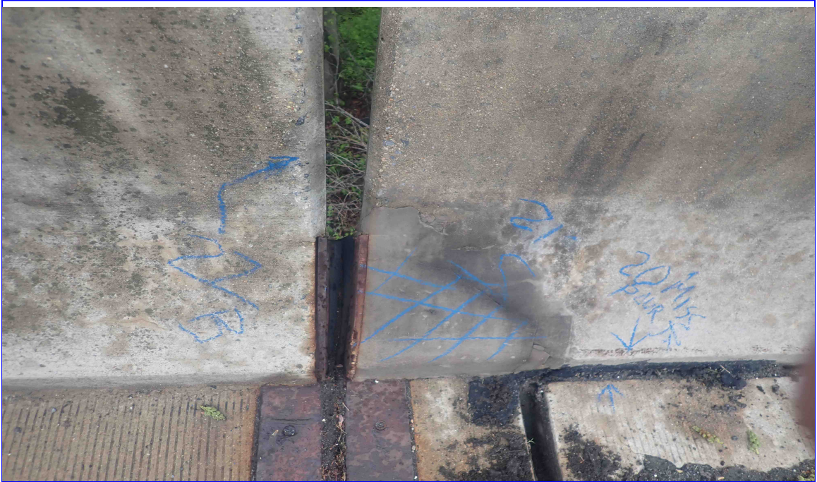
15. SPAN 1 S RC RAIL DELAM CURB PATCH ~22 FT FROM WEST END NORTH FACE LOOK S
