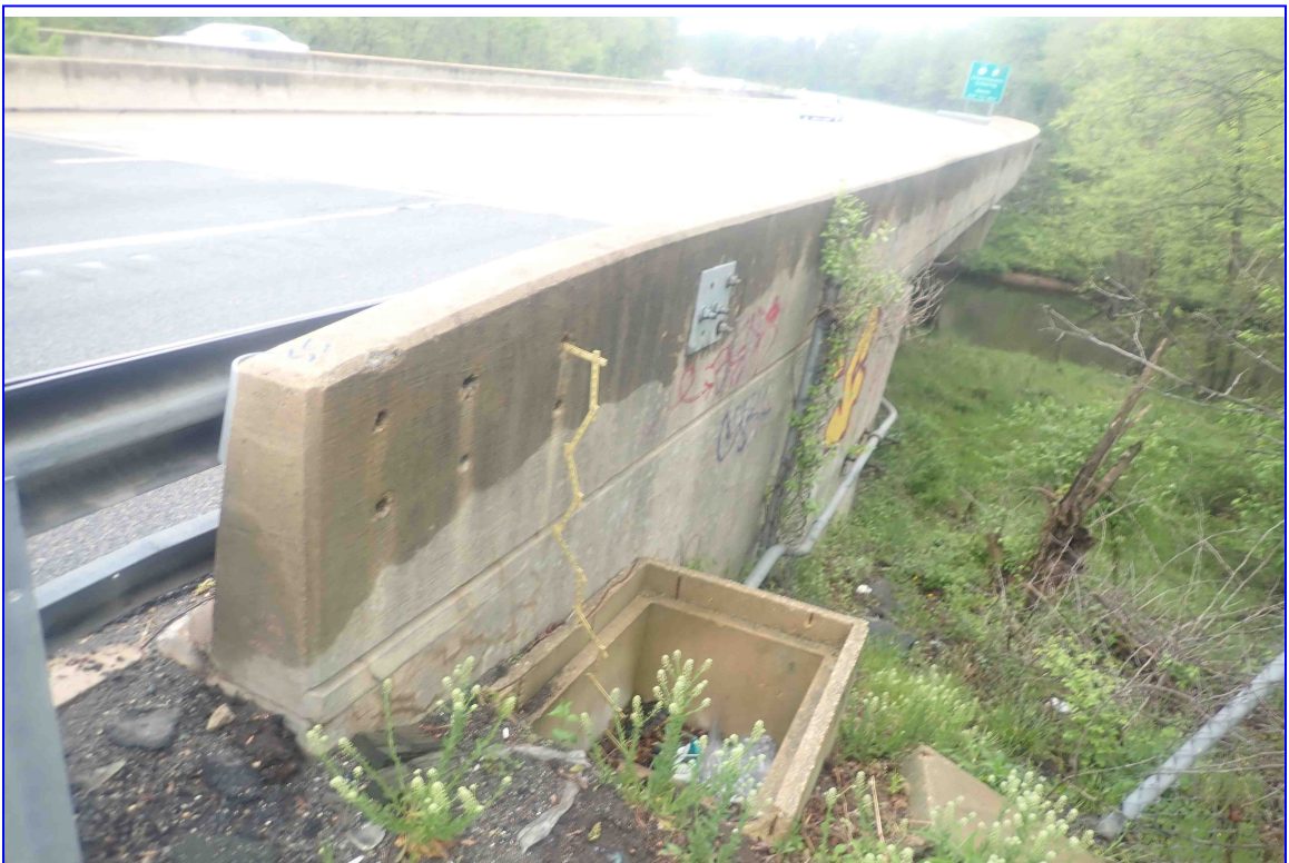
16. SPAN 1 S RC RAIL DEEP GUARDRAIL ATTACHMENT HOLES & OPEN UTILITY COVER LOOK E
