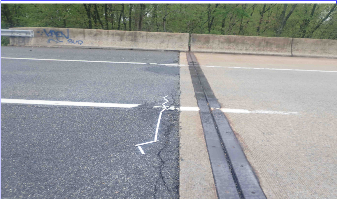
19. SPAN 3 E APPR SLAB LG ASPHALT WEARING SURFACE SPALLS & ~1/2 INCH CRACK LOOK S
