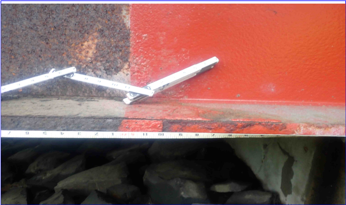
7. SPAN 1 N PAINT & WEATHR STEEL FACIA GIRDER 1 LAM CORROS AT W END LOOK S
