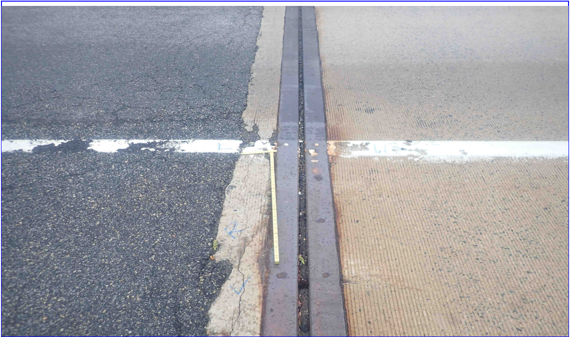
13. SPAN 1 STRIP SEAL HEADER SPALLS AT SOUTH SHOULDER & WHITE LINE LOOK N
