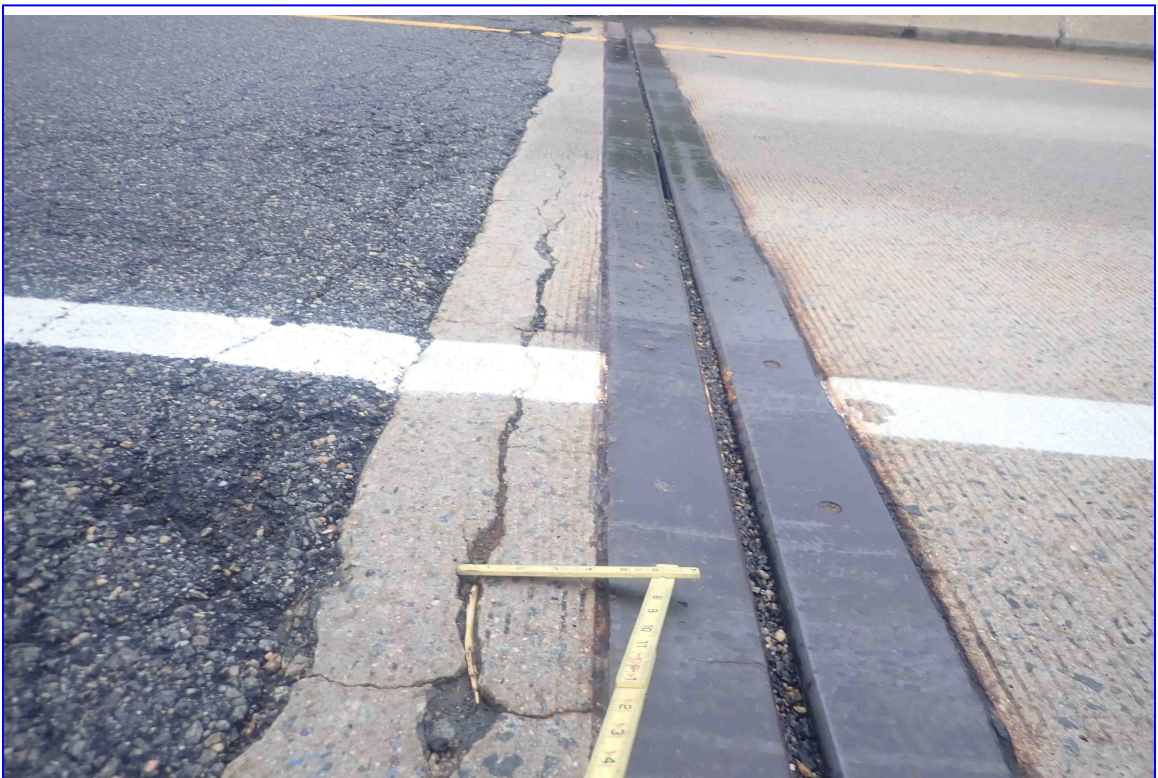
14. SPAN 1 STRIP SEAL W ABUT JOINT HEADER ~3/4 INCH WIDE CRACK AT CL RD LOOK N
