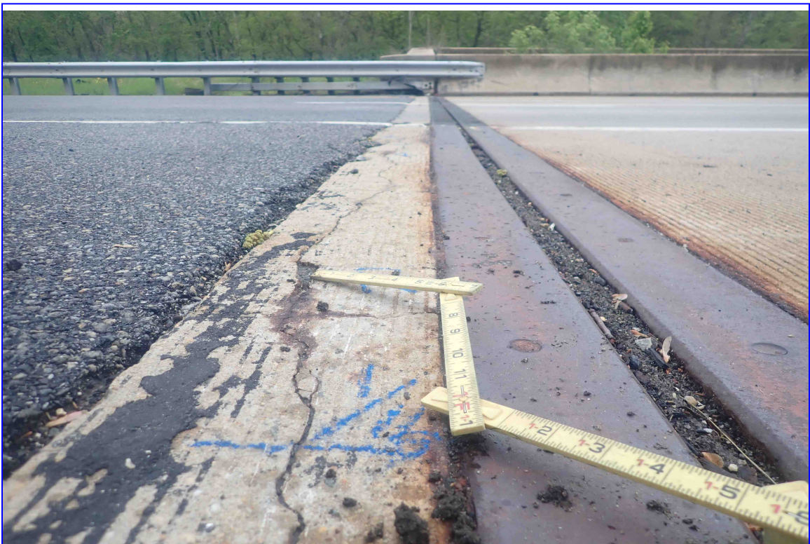
12. SPAN 1 STRIP SEAL HEADER RUST STAINED CRACK SOUTH SHOULDER LOOKING N
