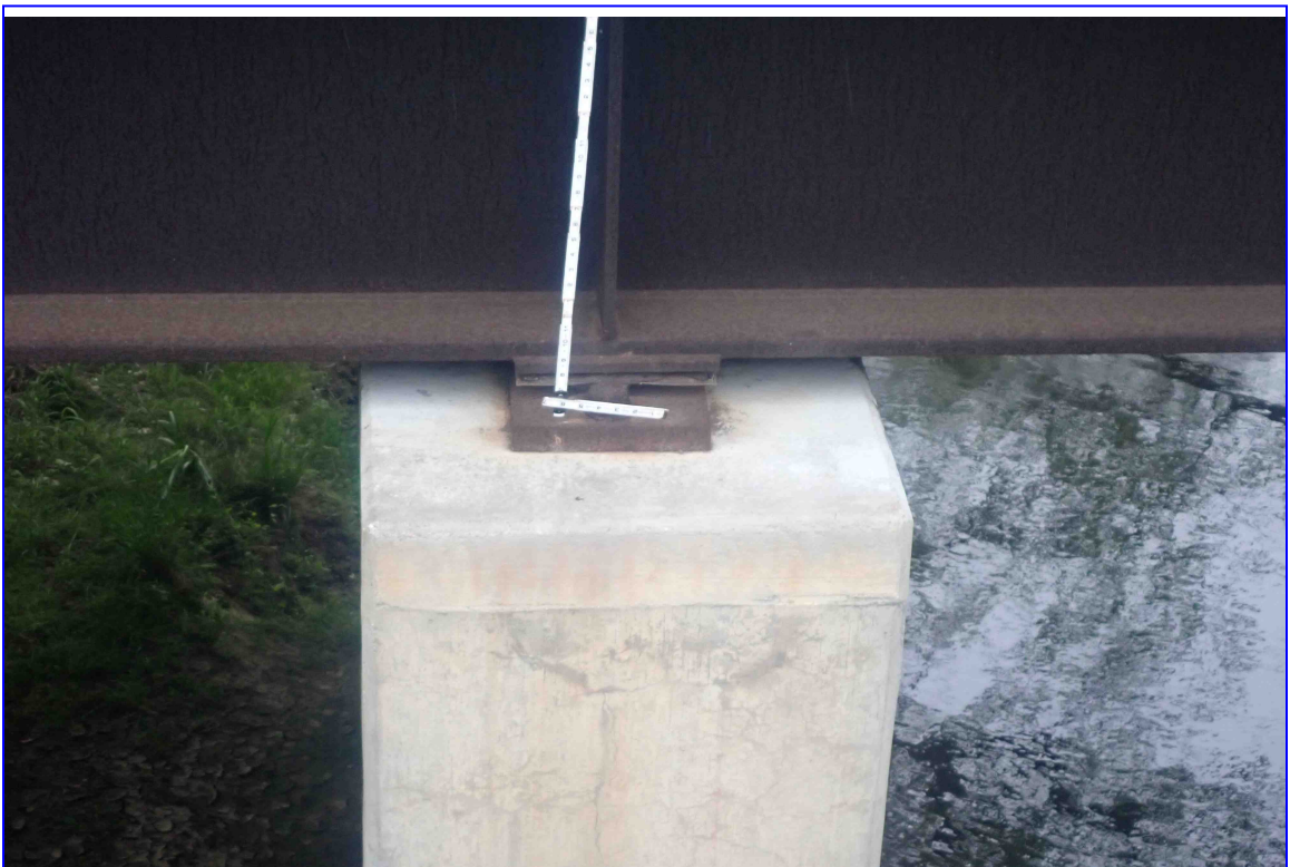
18. SPAN 2 PIER 2, N FACIA BEARING MISALIGN, TEPHLON PL SEPARATION & CORROS LOOK S
