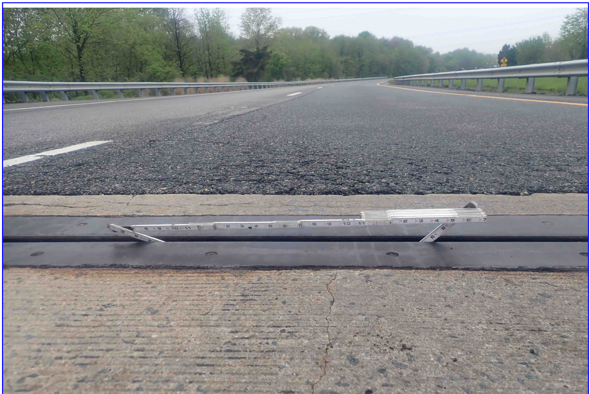
10. SPAN 1 STRIP SEAL JOINT GLAND PERFORATION ~28 FT FROM SOUTH END LOOK UP
