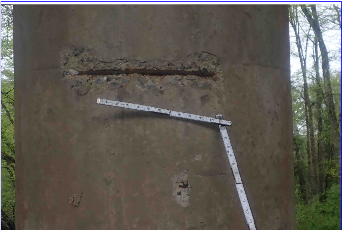
8. SPAN 1 WEST PIERWALL EXPOSED PITTED BARS AND SPALL AT NORTH END LOOK S
