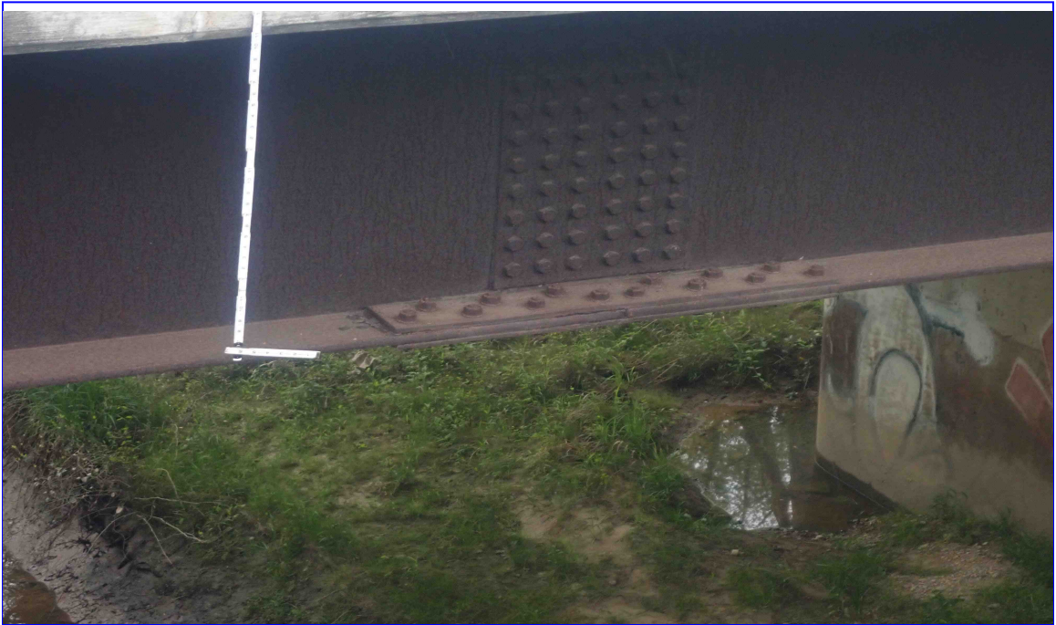
17. SPAN 2 N GIRDER SPLICE, CORROSION FLAKES & PACK RUST BETWEEN PLATES LOOK S
