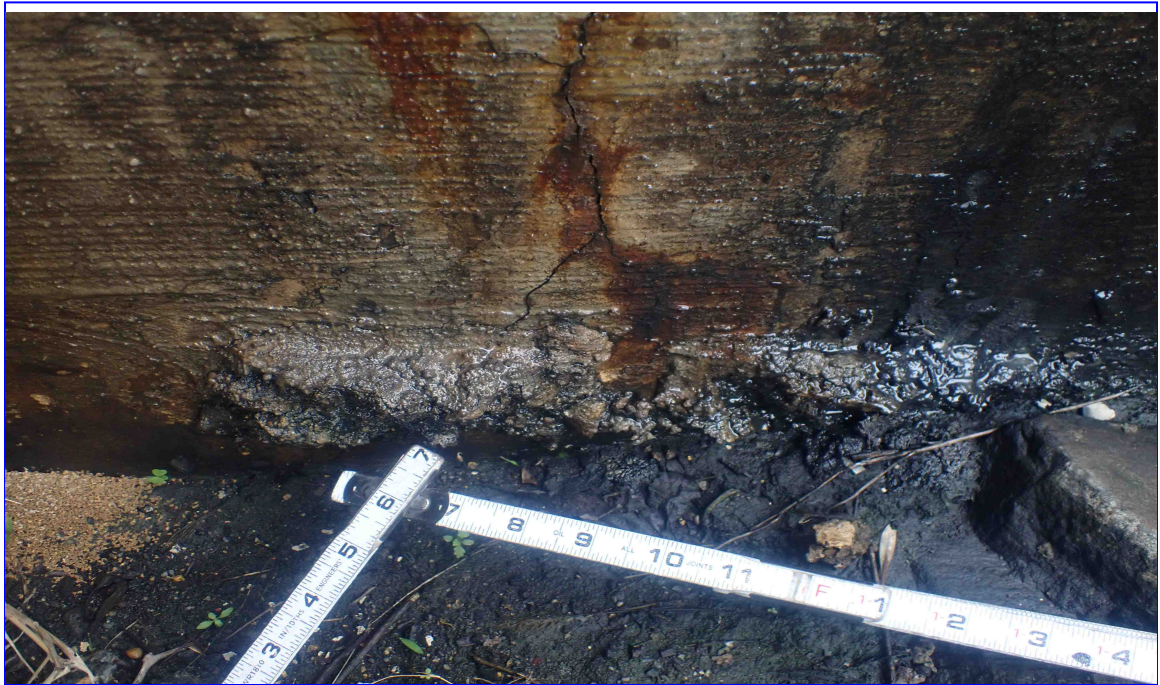
9. SPAN 1 W ABUTMENT STEM RUST STAINED CRACK ~43 FT FROM SOUTH END LOOK W
