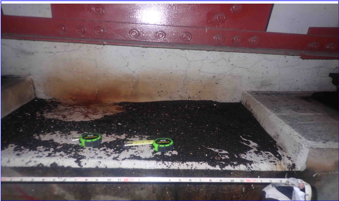
11. SPAN 1 STRIP SEAL JOINT IS LEAKING WATER & DEBRIS ON TOP OF W ABUT LOOK N
